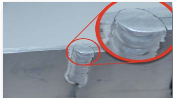
Weld Must Have Deep Penetration
